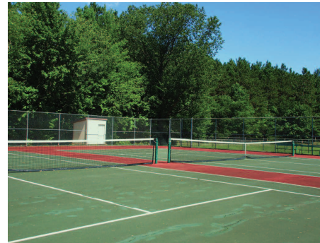
A network of patched and emerging cracks and dents in Boyne City's tennis courts at Rotary Park will be a thing of the past by next summer after new courts are installed. Once complete, the new tennis courts will feature painted markings to accommodate both tennis and pickleball players.
